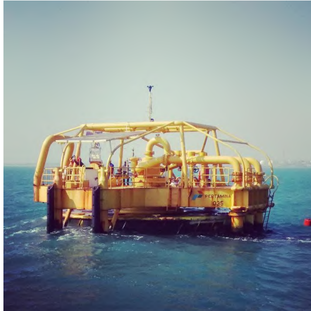
Gambar 1.1. SPM ( Single Point Mooring ) 035 Pertamina TBBM Tuban (Dokumen Pribadi)
