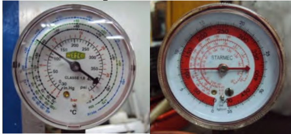
Gambar 3.14 High-low pressure gauge
