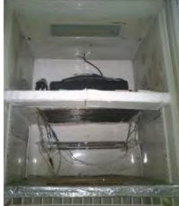
Gambar 3.7 Evaporator Low stage
