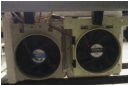
Gambar 3.6 Display Cooling water box
