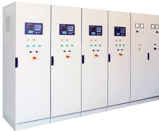
Gambar 2.10. Gambar Panel Sinkron
