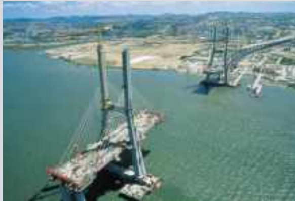
Vasco da Gama Bridge, Portugal with fuse box for earthquake movements built: 1997 Cable-stayed bridge main span: 829 m type of joint: DS1440 59.00 lin. metres
