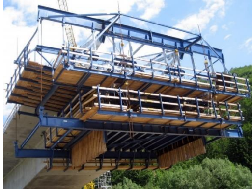
Gambar 4.13 Form traveler milik Handan China Railway Bridge Machinery Co.Ltd
