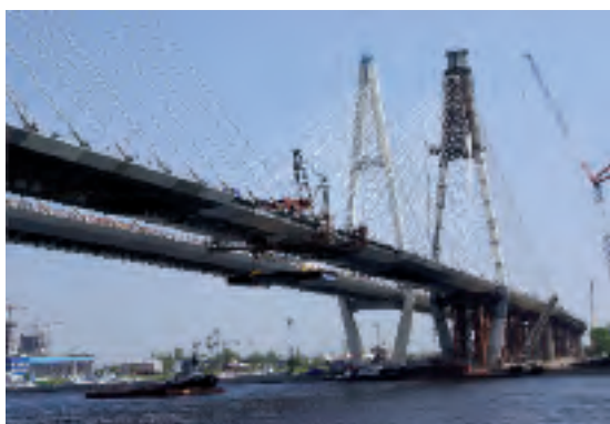
Neva 2 Bridge, Russia (2007) Supply and installation of stay cables with VSL Friction Dampers
