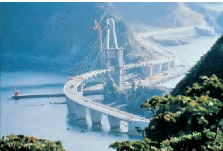
Koshiki Daimyojin Bridge, Japan (1993) Technical consultation and supply of the prefabricated stay cables
