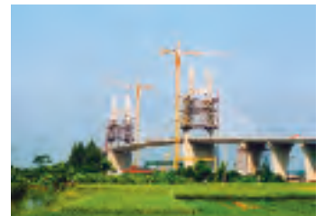
Kien Hai Phong Bridge, Vietnam (2003) Supply and installation of bearings and stay cables
