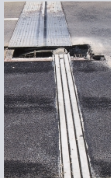
Replacement of a Roller Leaf Joint by a MAURER Swivel Joist Expansion Joint
