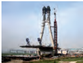
Taipei Ring road Bridge, Taiwan (2009) 13 pairs of stays on each side of the pylon
