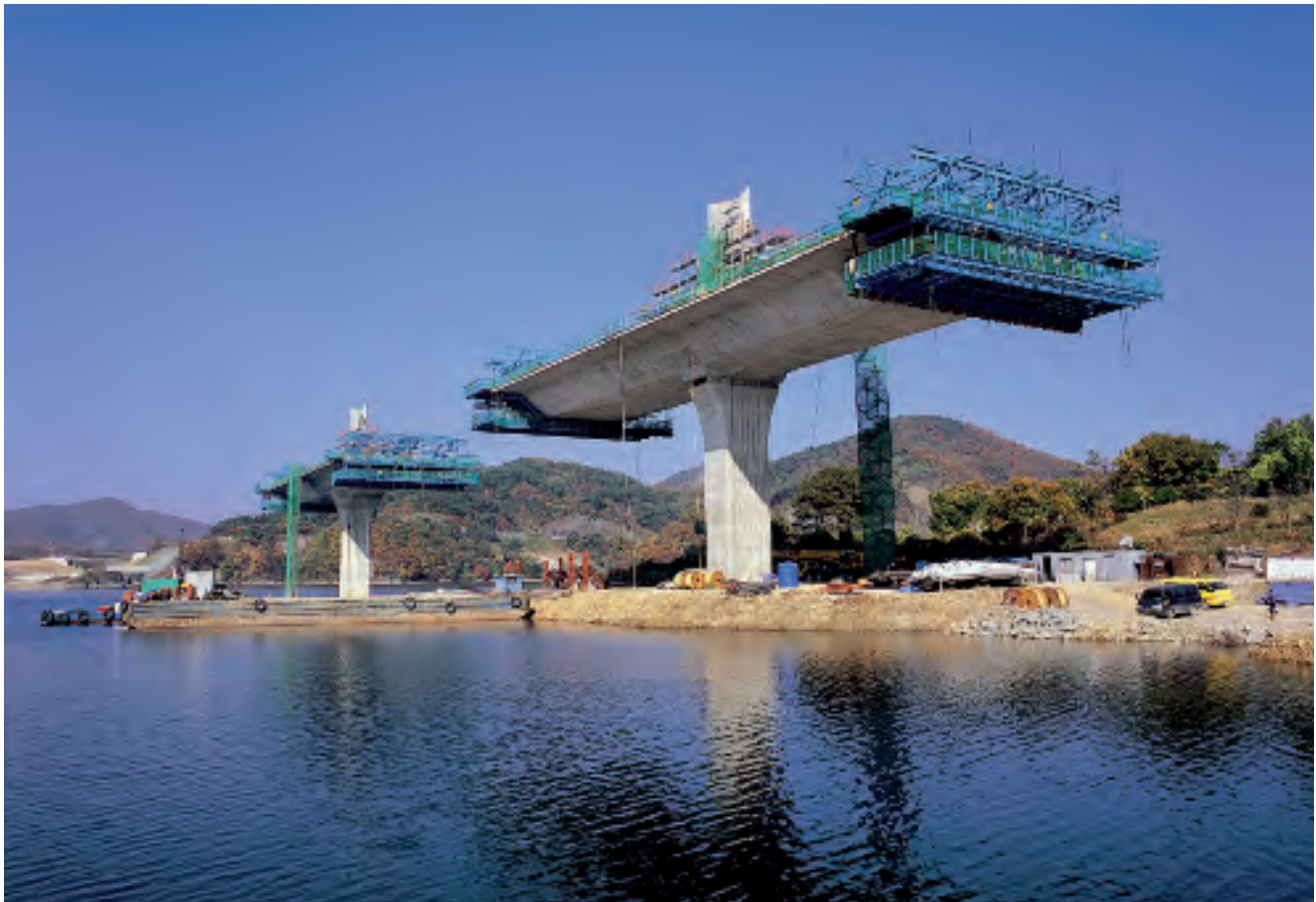
Woonam Bridge, South Korea (2008) VSL pylon saddles designed to allow cable replacement
