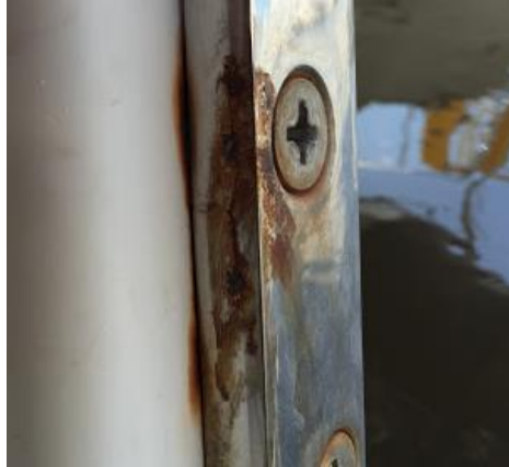
Gambar 2.3 Crevice Corrosion (Sumber : dirigomaritime.com )
