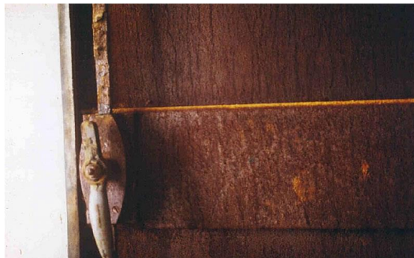
Gambar 2.1 Korosi Homogen (Sumber : cdcorrosion.com )
