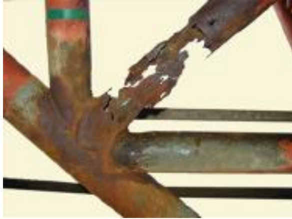
Gambar 2.6 Fatigue Corrosion (Sumber : Askitians.com )
