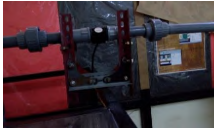
Gambar 3.6 Pemasangan 1" Water Flow Sensor
