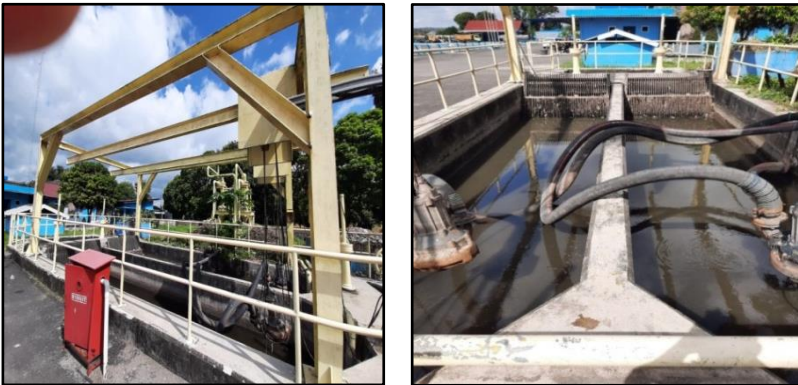
Gambar 4.2 Unit Grit Chambers
