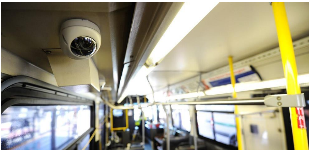
Gambar 2. 18 CCTV mumbai (Sumber : The Urban Vision hal.25)
