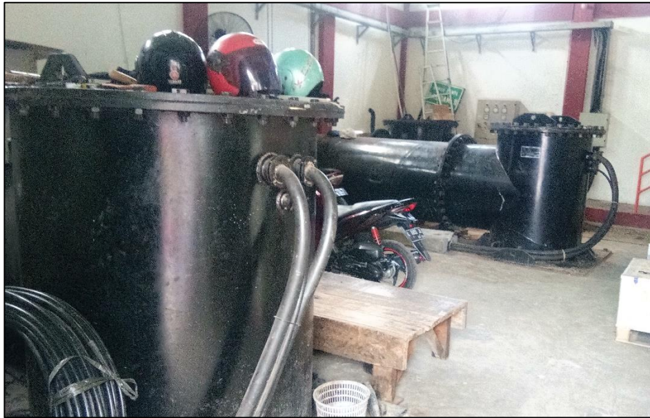
Gambar 4.7 Pompa Air Boezem Kalidami
