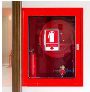
Gambar 4.25 Fire Hydrant Sumber: Google.com (2020)
