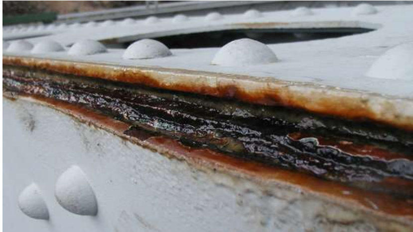
Gambar 2.5 Contoh tipe Crevice Corrosion
