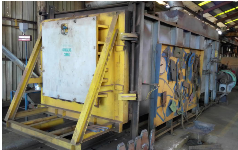
Gambar 8.1. Unit Burner – Annealing Furnace Car Type
