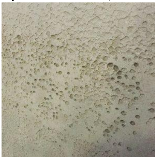
Figure 4- 16 Pitting Corrosion Inside a Storage Tank (Source: abfad.co.uk)
