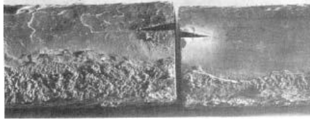
Gambar 2. 8 Superheater Tube yang Pecah Akibat Coal Ash Corrosion. (Port, Herro and Robert, 1991)
