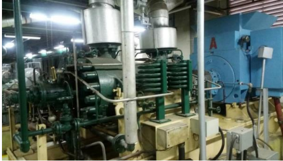
Gambar 4.2 High Pressure Boiler Feed Pump PLTGU PT X
