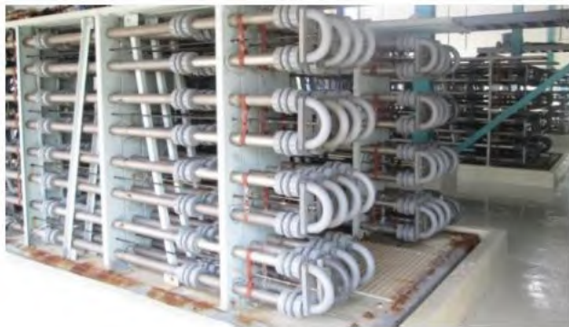
Gambar 4.10 Sistem Klorin di PJB UP Gresik (Rendal Operation PLTU PT. PJB UP. Gresik)
