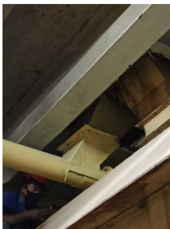
Instalasi Screw Conveyor PT. Sreeya Sewu
