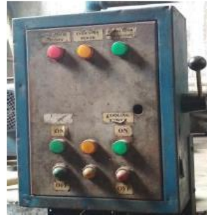
Gambar 2.4 Main water in atau control Water in .
