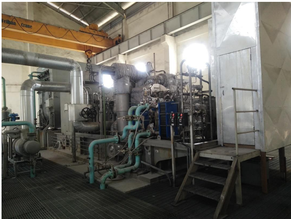
Gambar 2.4 Steam Turbine Generator 17.5 MW di Petrokimia Gresik II
