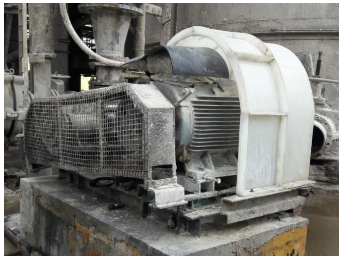
Gambar 5. 1 Pompa Dihydrate Slurry P 2401 A
