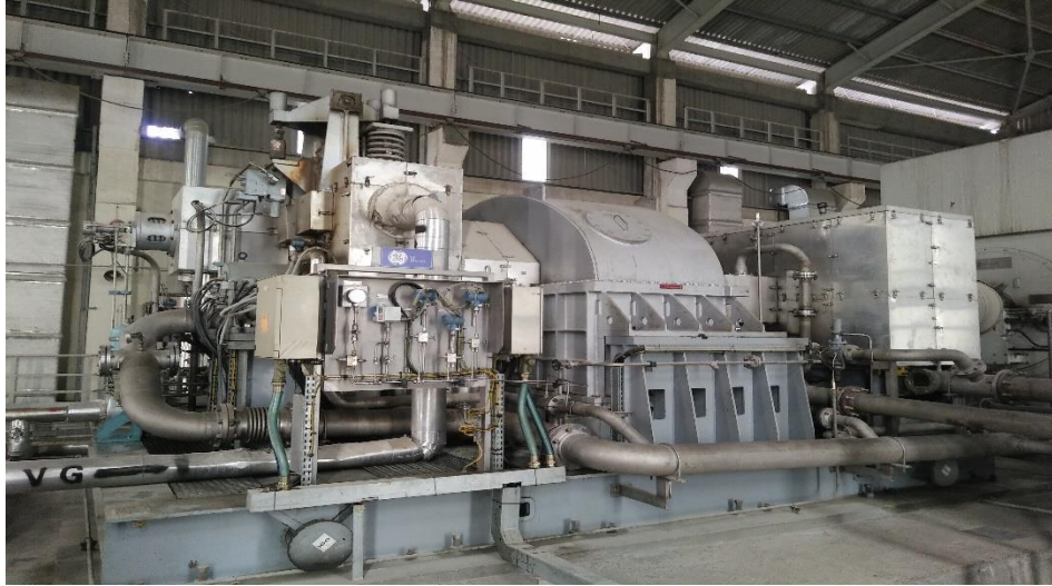
Gambar 2.2 Steam Turbine Generator 17.5 MW di Petrokimia Gresik
