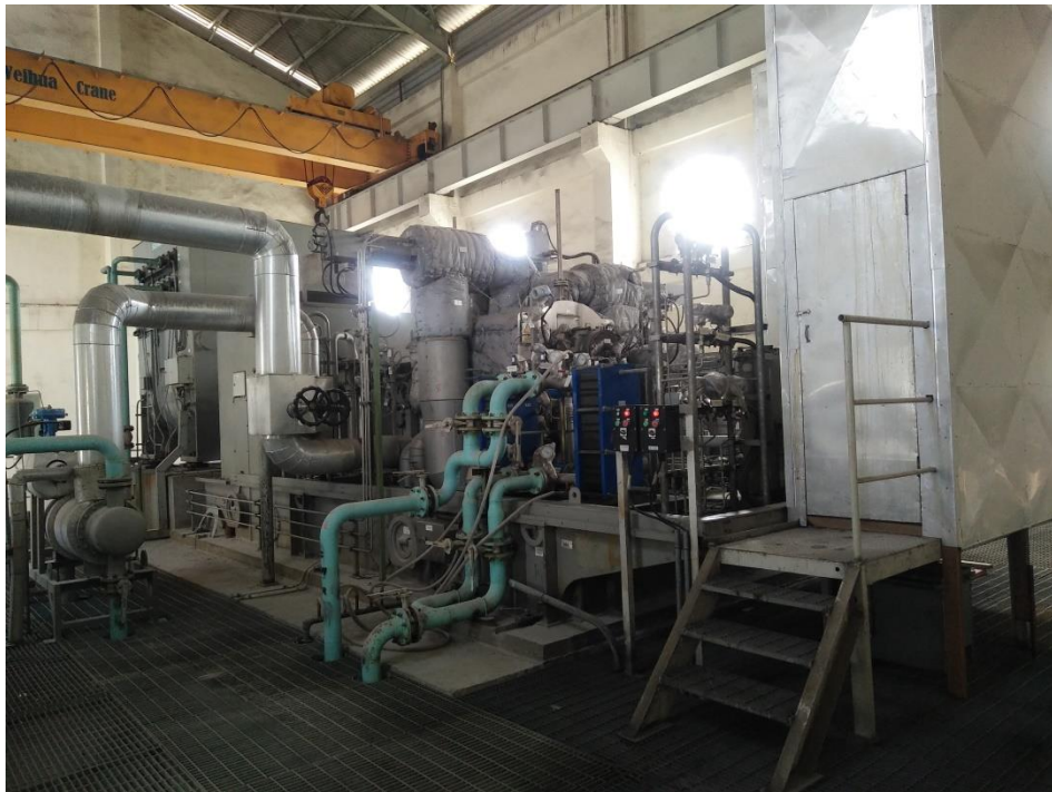
Gambar 2.3 Steam Turbine Generator 12.5 MW di Petrokimia Gresik
