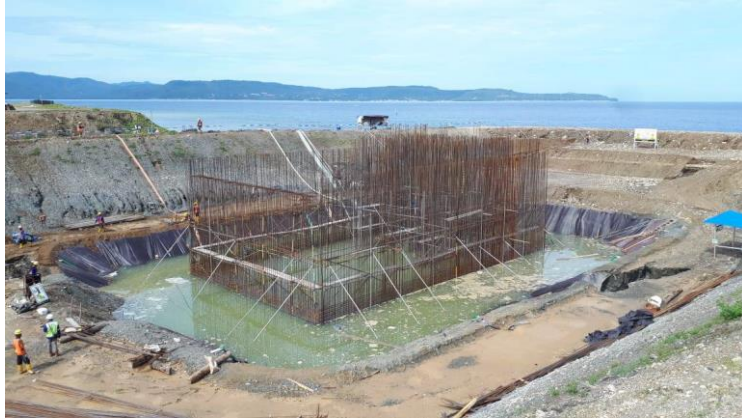
Gambar 8 1 Pump House Terendam Air Laut
