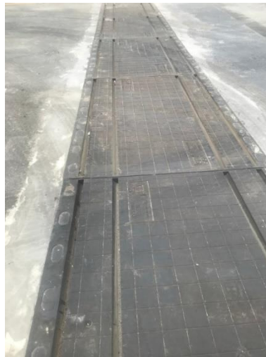
Gambar 4.13 Hasil akhir pekerjaan seismic expansion joint jembatan SB Arch Ahmad Yani P346
