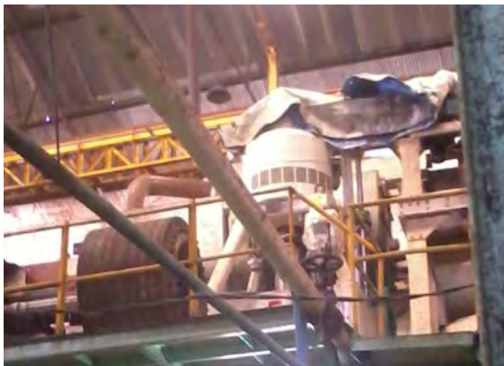
Gambar 2.11. High Grade Fugal (HGF)
