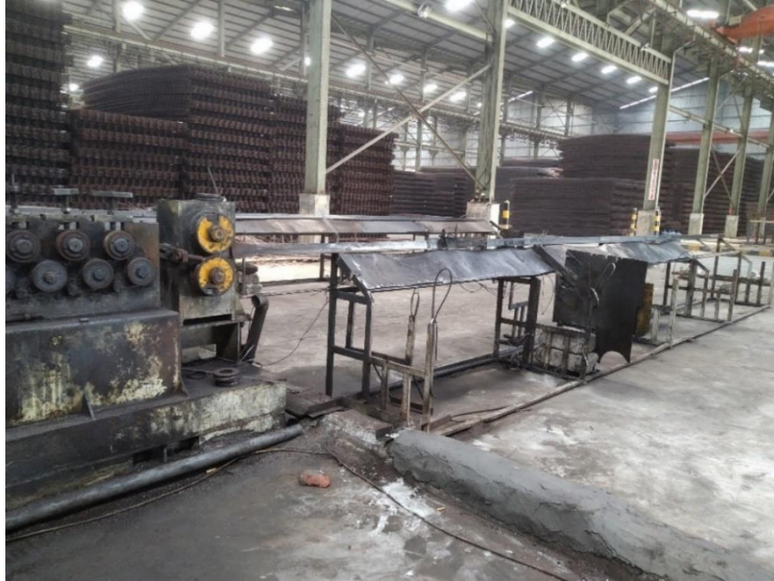
Gambar 4.17 Cold Ribbed Wire Plant Bagian Belakang
