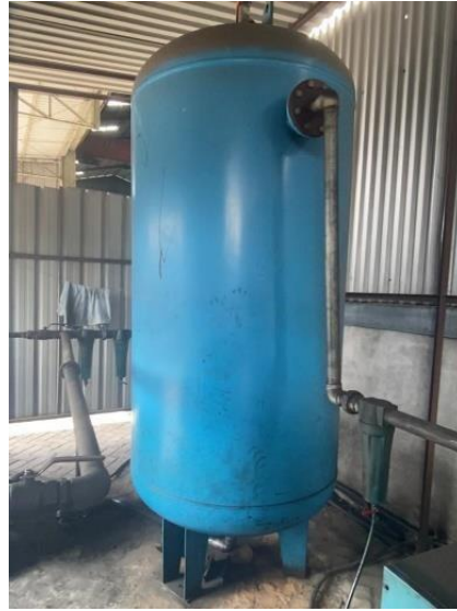
Gambar 4.42 High Pressure Air Receveir Tank
