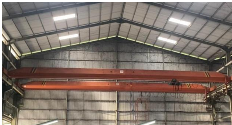
Gambar 4.43 Overhead Crane Single Girder
