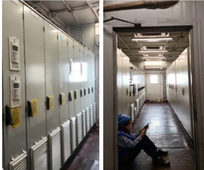
Gambar 4. 26 Electric Room CC 04
