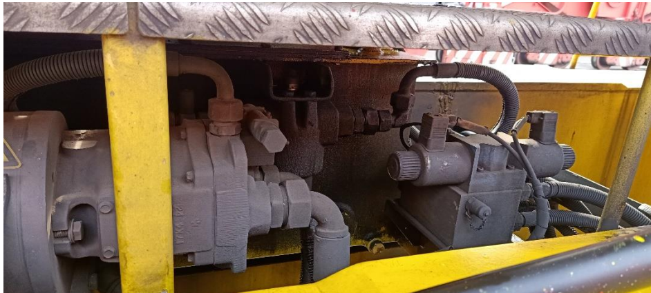
Gambar 4. 63 Power Pack Spreader Container Crane 05
