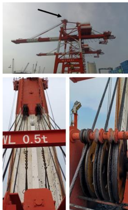
Gambar 4. 27 Pylon Containe Crane (CC) 05
