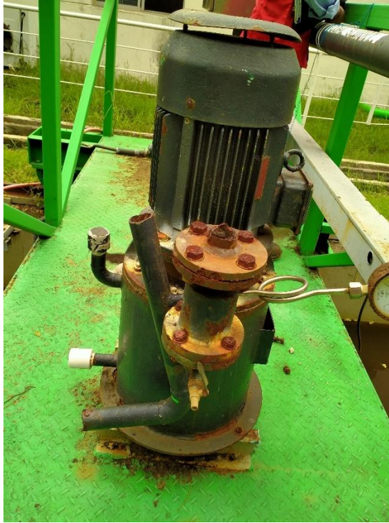
Gambar 4.36 Kondisi Motor Mud Suction Pump
