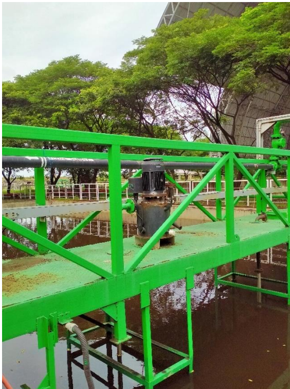
Gambar 4.37 Bridge Crane Sludge Scrapper
