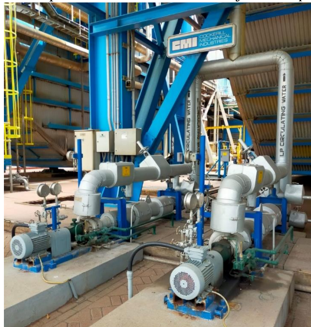
Gambar 4.11 Low Pressure Boiler Circulating Pump PLTGU
