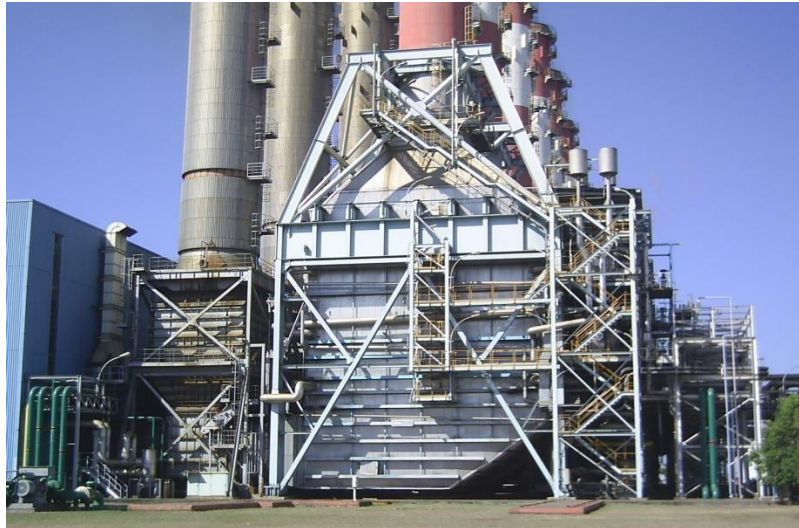
Gambar 4.6 Heat Recovery Steam Generator
