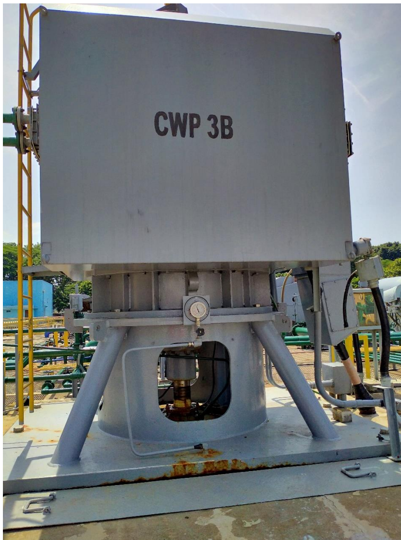
Gambar 4.26 Circulating Water Pump
