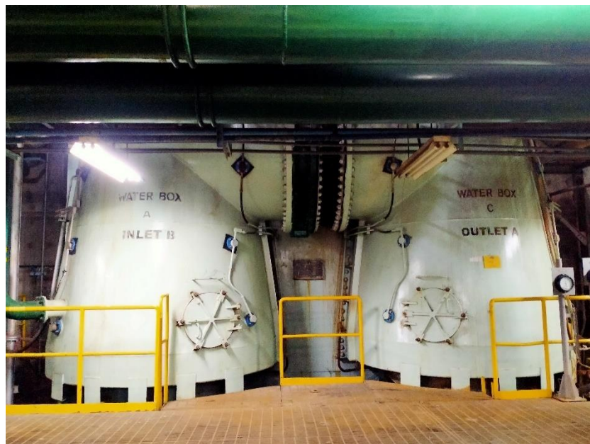
Gambar 4.23 Water Box Kondensor
