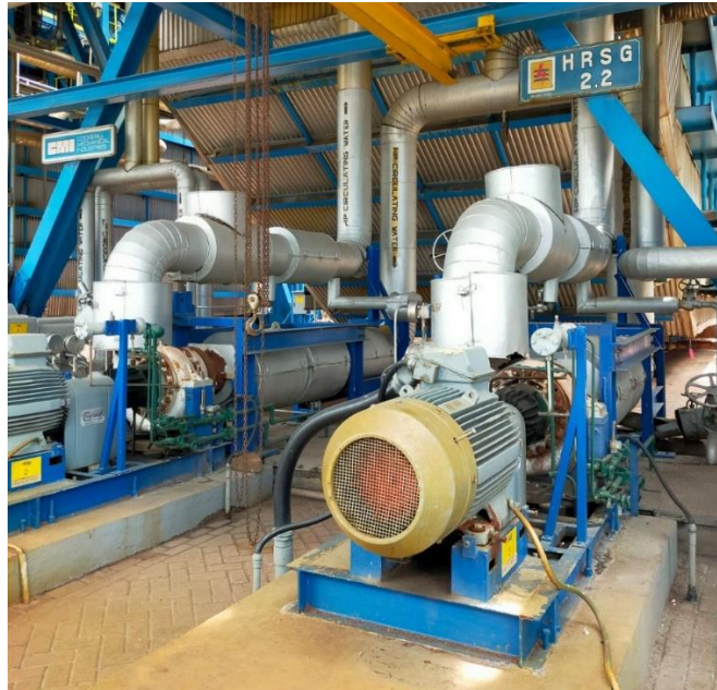
Gambar 4.12 High Pressure Boiler Circulating Pump PLTGU
