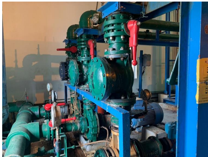
Gambar 4.17 Sea Water Booster Pump
