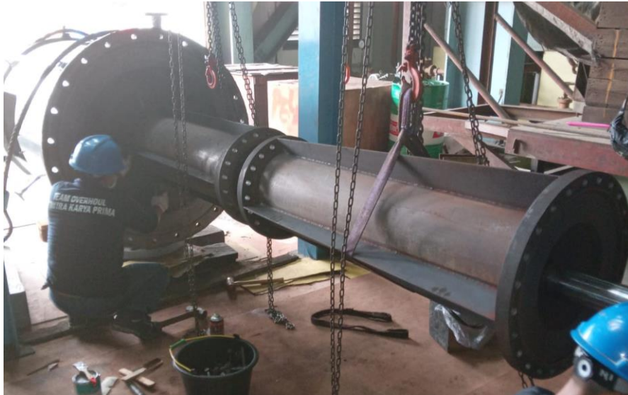
Gambar 4. 27 Condensate Extraction Pump
