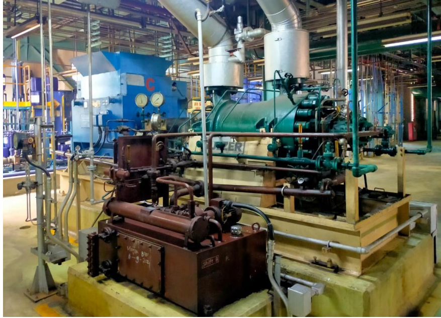
Gambar 4. 26 HP Boiler Feed Pump PT. PJB UP Gresik
