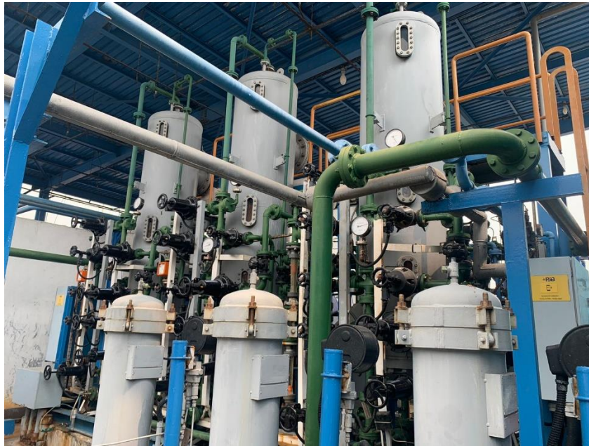
Gambar 4. 12 Water Treatment Plant
