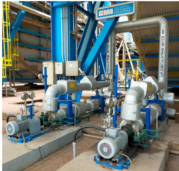
Gambar 4. 22 LP Boiler Circulation Pump (PJB Gresik)
