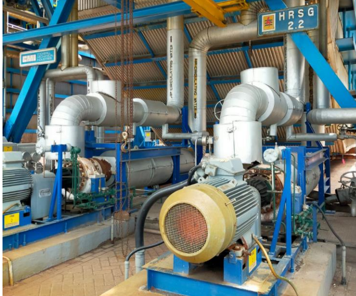
Gambar 4. 24 HP Boiler Circulation Pump (PJB Gresik)
