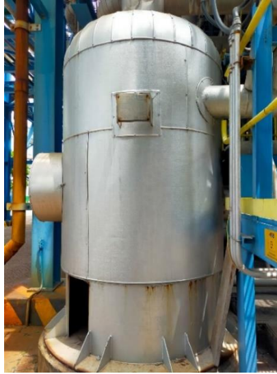
Gambar 4. 29 Brine Blowdown Tank
