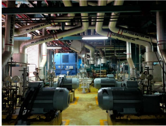
Gambar 4. 25 LP Boiler Feed Pump PT. PJB UP GSK
