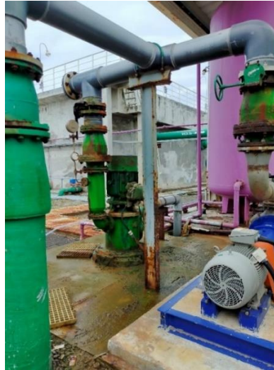
Gambar 4. 25 Slurry Transferring Discharge Pump
